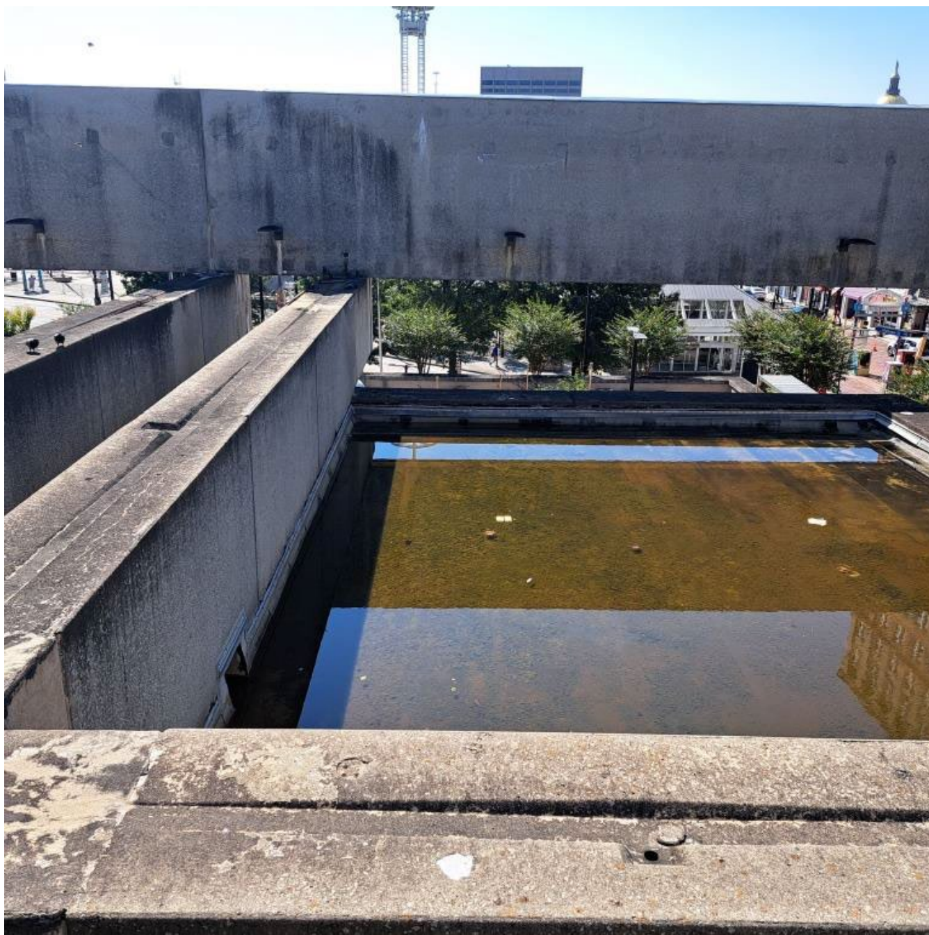
FIGURE 7. WATER RETENTION ON FLAT ROOF
