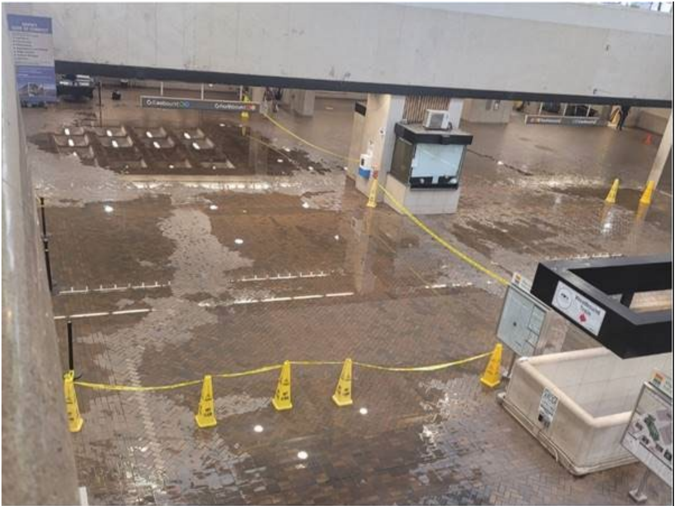
FIGURE 5. EXAMPLE OF WATER CONDITIONS ON THE CONCOURSE LEVEL AFTER A STORM EVENT
