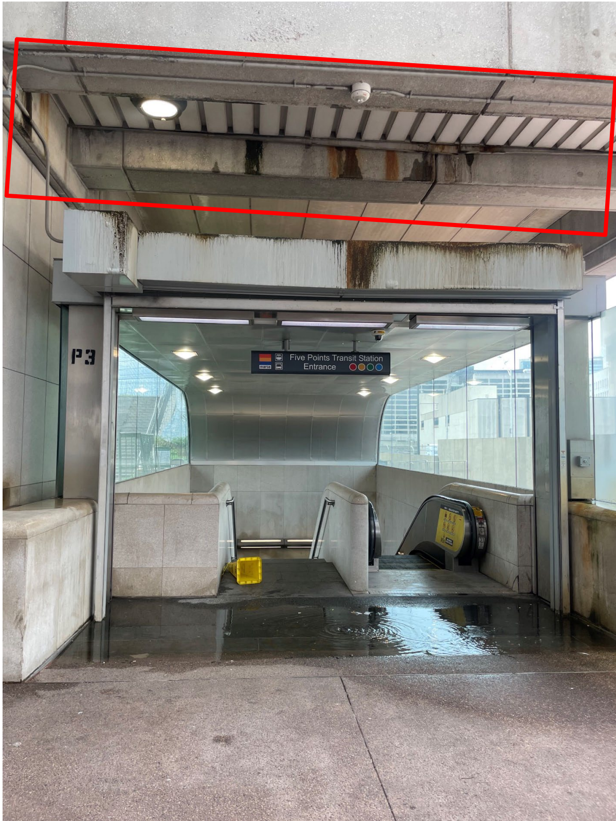
FIGURE 6. EXAMPLE OF THROUGH LEAKING DAYS AFTER A STORM EVENT THAT IMPEDES STATION MOBILITY
